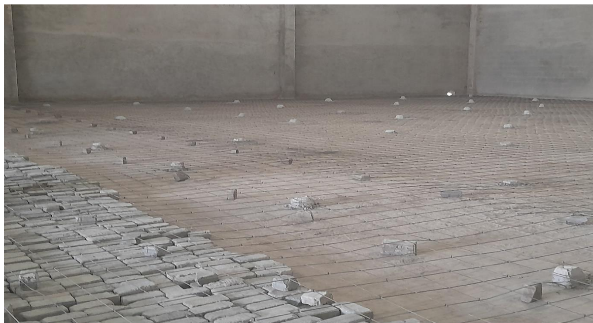
Picture of stalled works
